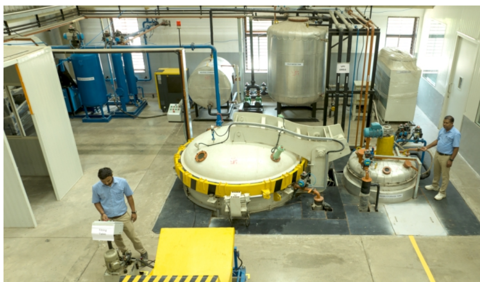
Vacuum Impregnation Plant
